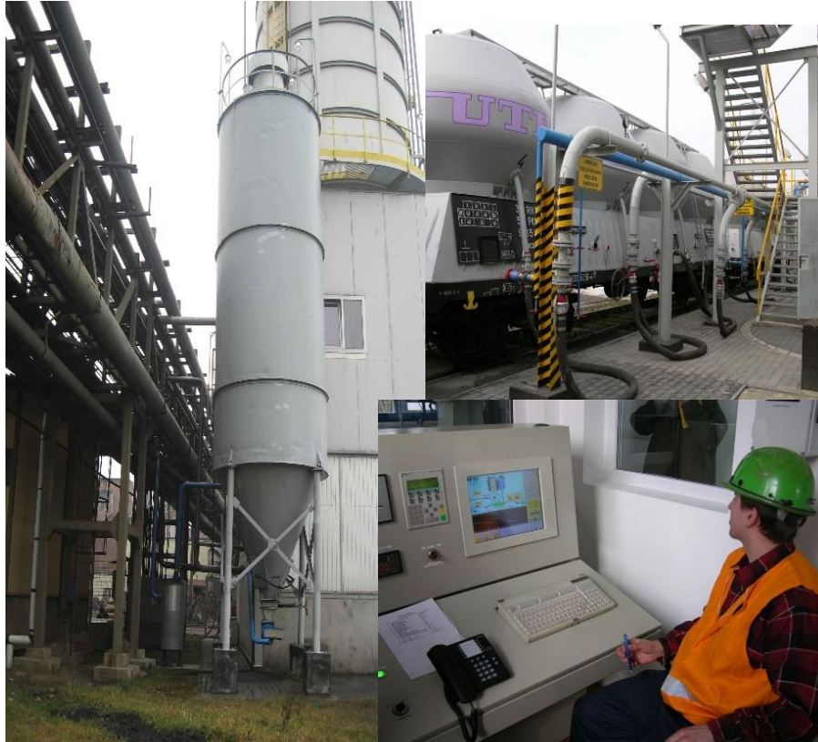
Figure 3. Fly ash – water slurry preparation plan at “Szczygłowice” mine. On the left: fly ash tank and main building behind binder tank, right up: pneumatic fly ash discharge from tank wagon. Right down: control room (Palarski et. al., 2011)
